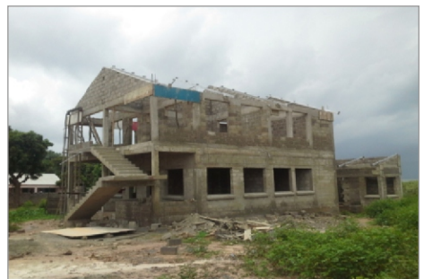
Construction of New Staff Housing at Farafenni Hospital in North Bank Region
