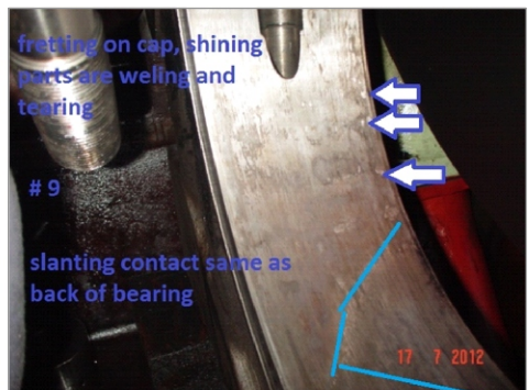
ECOWAS EMERGENCY POWER SUPPLY PROGRAMME
