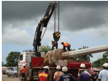
Energy Transmission & Distribution (LEC)
