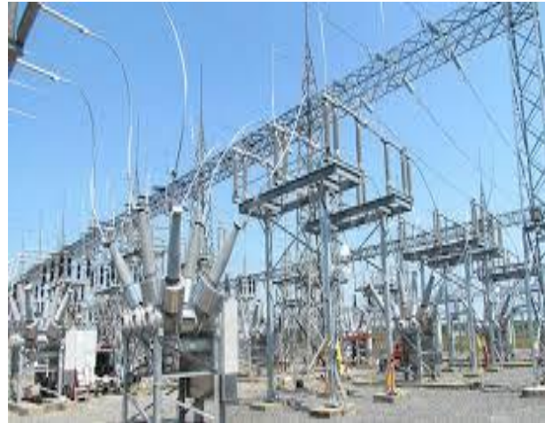
33 MVA Transformers at Mim in the Western Region
