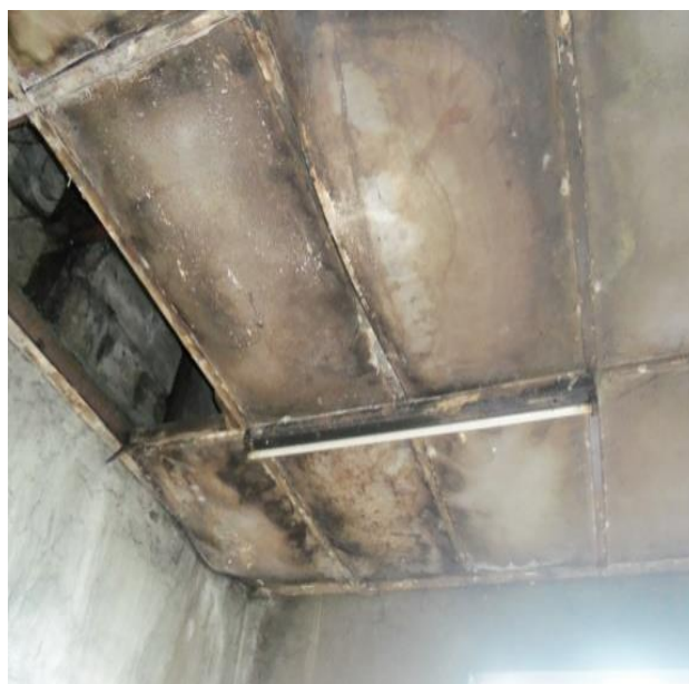
Figure 1 - Damaged Roof at Central Medical Stores
